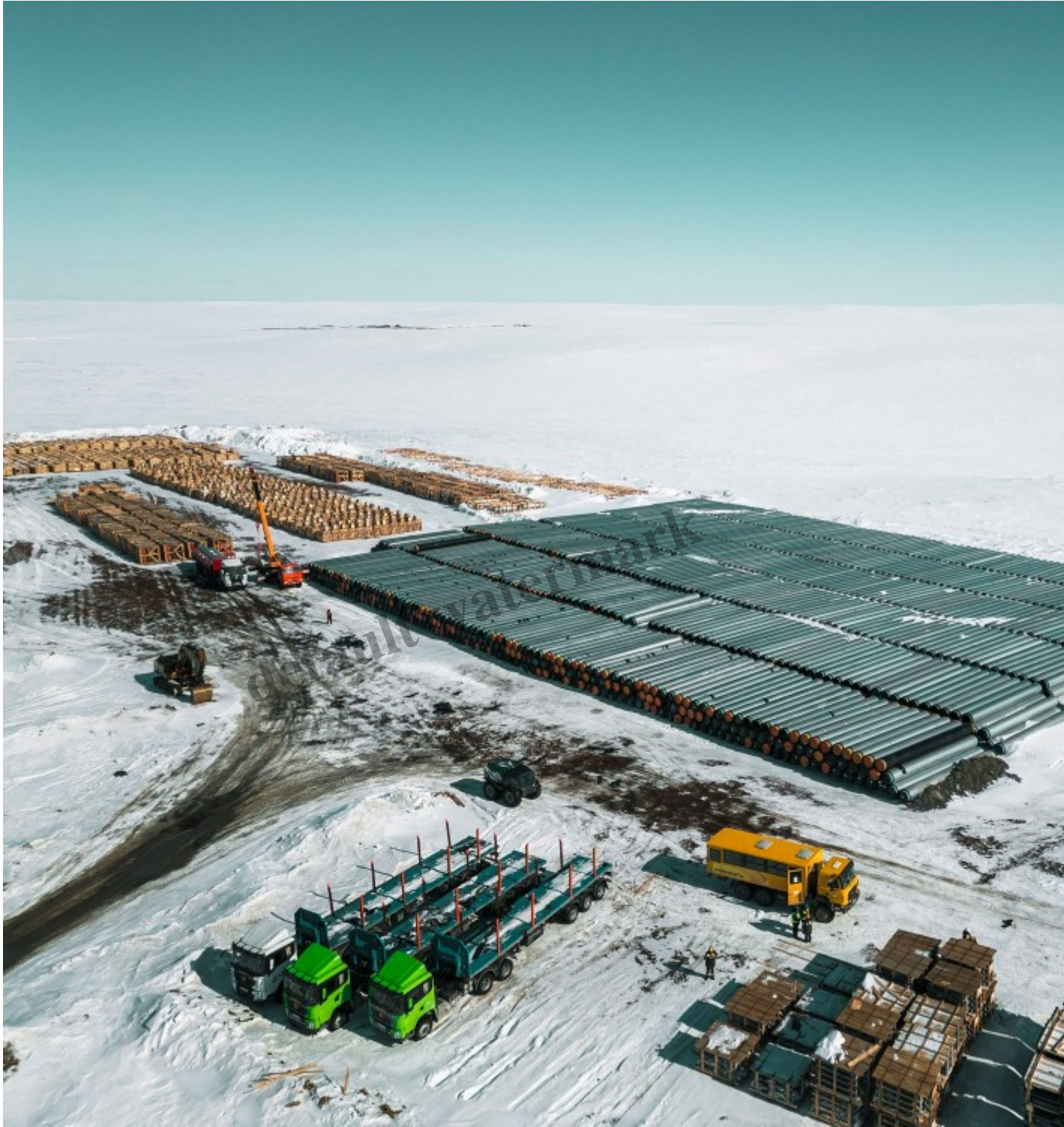
At least 21 km of oil pipes stacked along the shores of the Yenisey River ready to be assembled as part of pipeline (VK)
